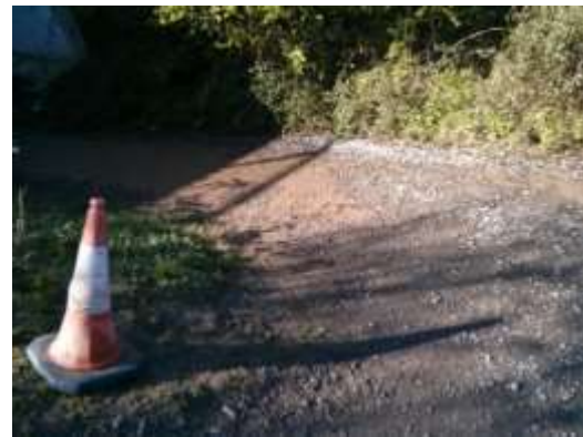
Steep slope with chippings which can puncture tyres - NCN41 underpass under A40
