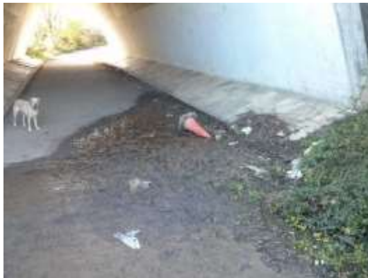
Flooding in NCN41 underpass under A40
