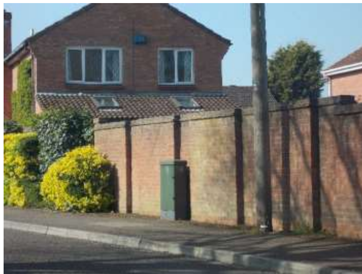
Good use of brick at side of property, robust, has endured well, Bader Avenue Estate, Churchdown
