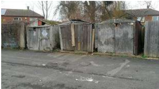
Dilapidated garages at Swallow Crescent, Innsworth
